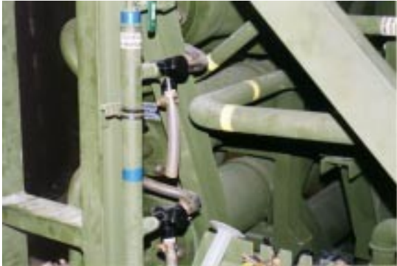
Figure 36. Rear R.O. Pressure Tube Vent/Sample Valves.
