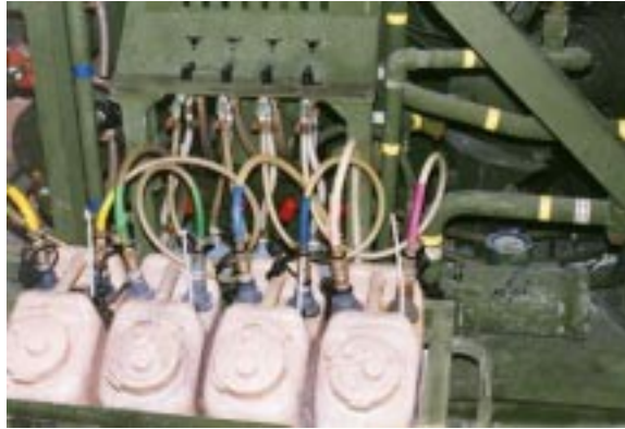
Figure 30. Chemical Feed Can Connections.
