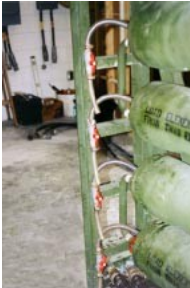
Figure 35. Front R.O. Pressure Tube Vent/Sample Valves.
