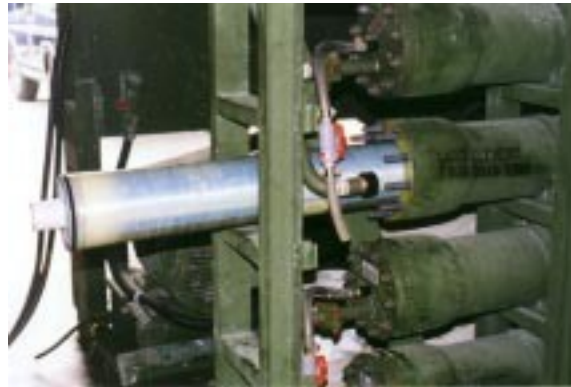
Figure 51. Insertion of R.O. Element into Pressure Tube.
