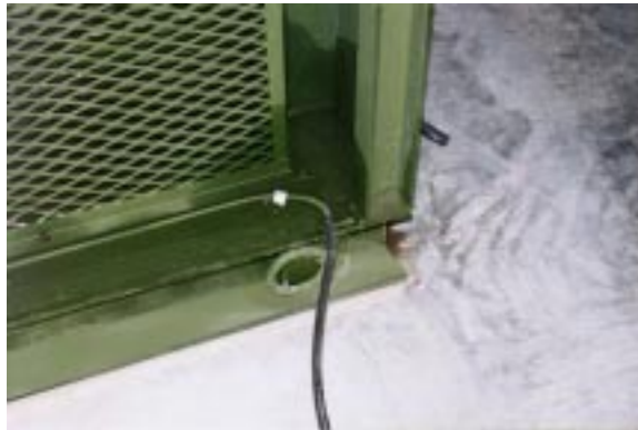
Figure 39. Vent Pipe for the Three Vent Valves.
