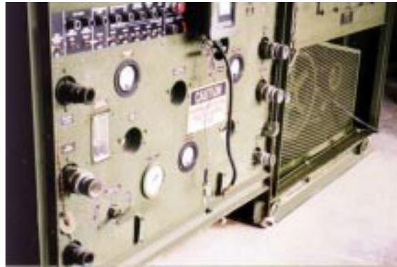
Figure 21. Quick Disconnect Fittings on Control Panel.
