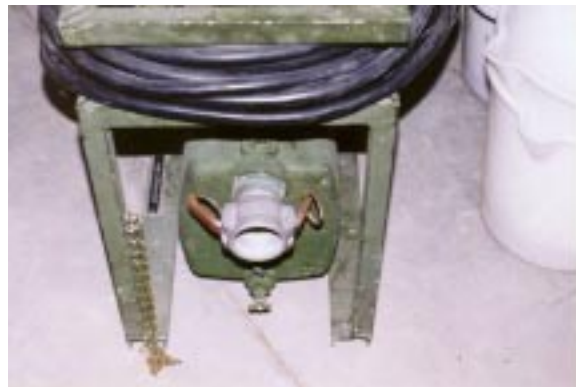
Figure 22. Fittings Attached to Raw Water Pump #1.
