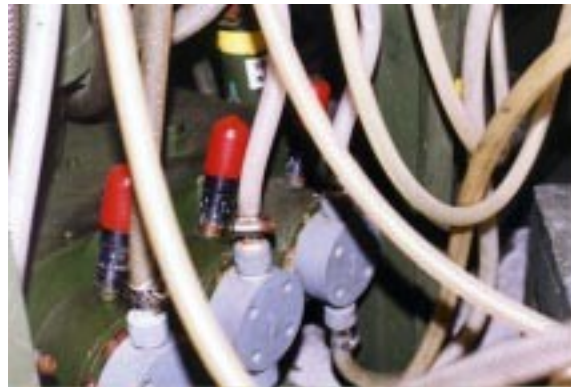
Figure 38. Chemical Feed Pump Controls.
