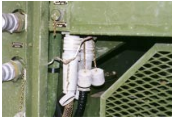
Figure 31. Electrical Power Connections at Junction Box.
