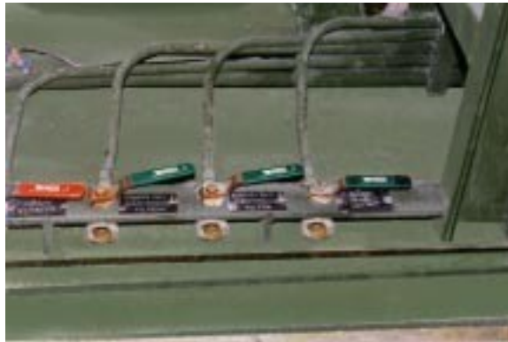
Figure 42. Cartridge Filter Drains #1 and #2.
