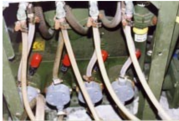
Figure 9. Chemical Feed Pump.
