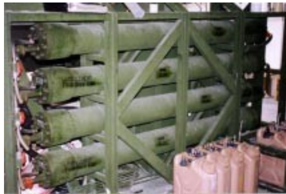
Figure 2. Reverse Osmosis Pressure Tubes.
